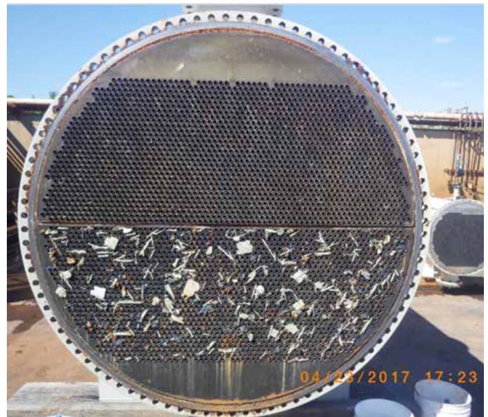
Figure 2. Debris in the inlet of critical heat exchanger.
